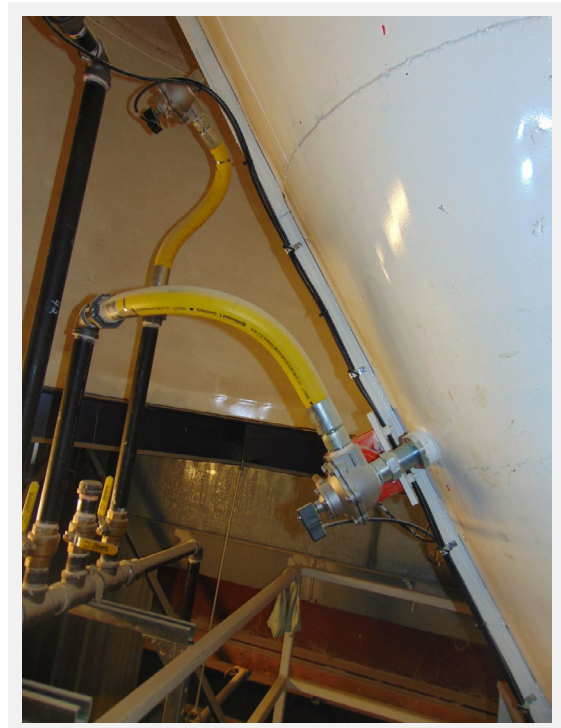
Strategically-positioned VA-12 units on dry-mix bin
